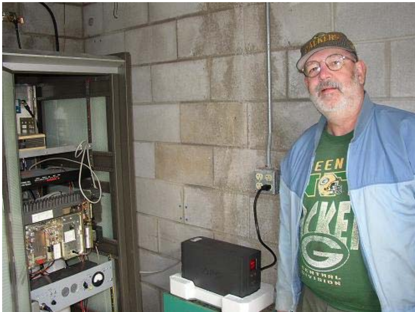
KDØCI stands by the newly installed Ogilvie Repeater UPS Backup Power Supply. [Photo by KDØFLQ]
