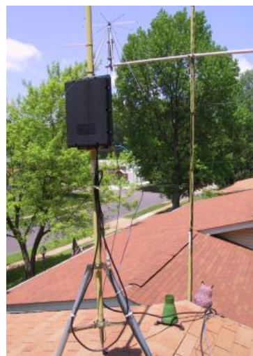
The SG-230 antenna coupler in its initial position, just above the roofline.
